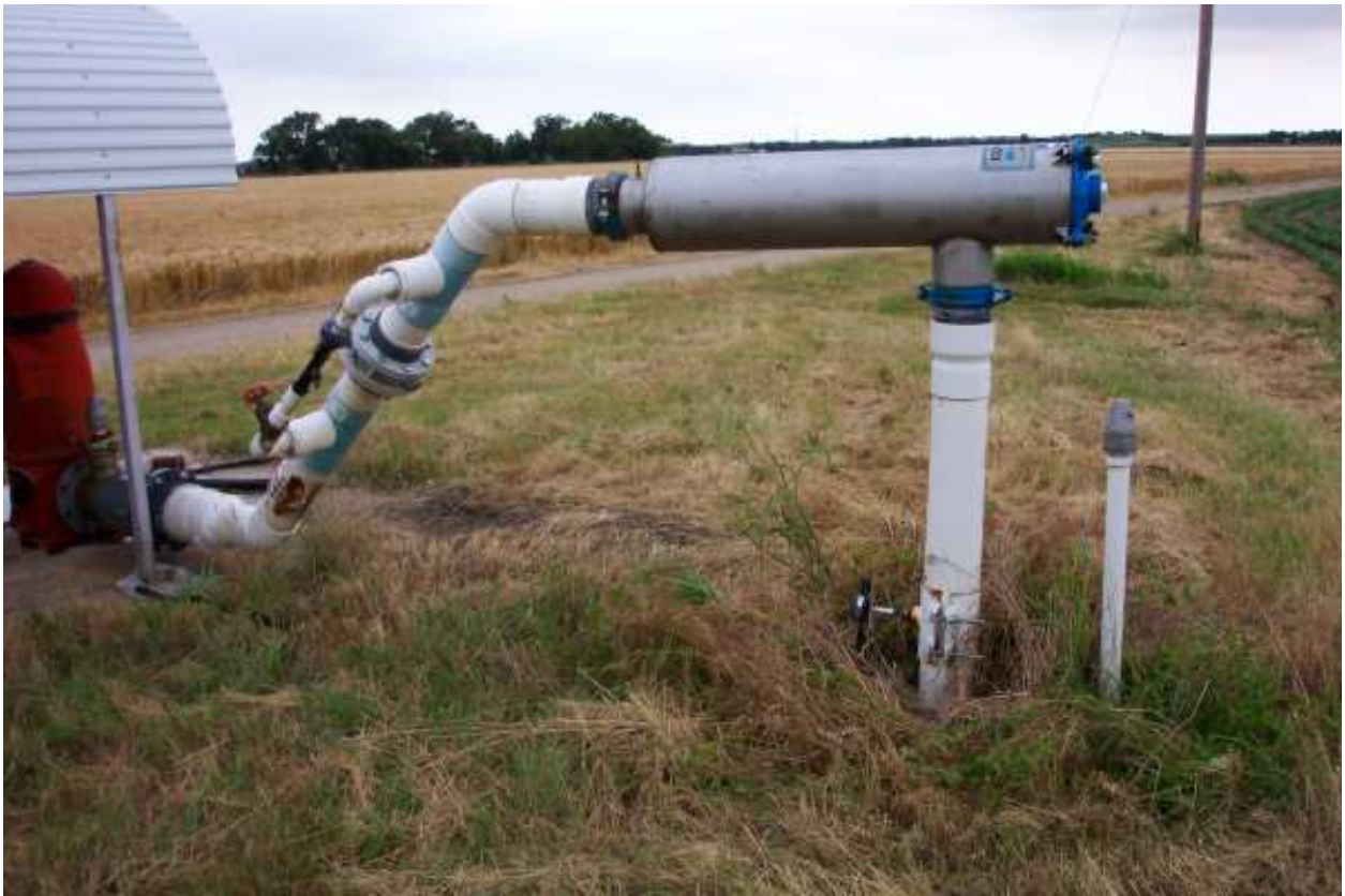
Figure 3a: Original pumping plant and filtration configuration of the case study SDI system.
