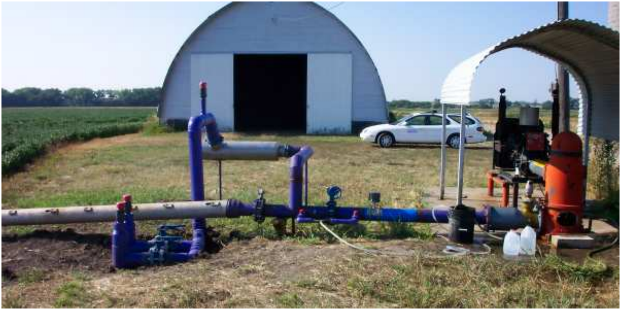
Figure 3b. Improved pumping plant and filtration configuration of the case study SDI system.
